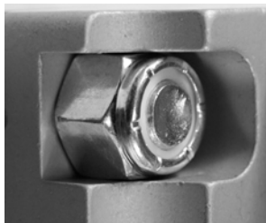
Fig 21 Bolt protrudes just beyond flush
